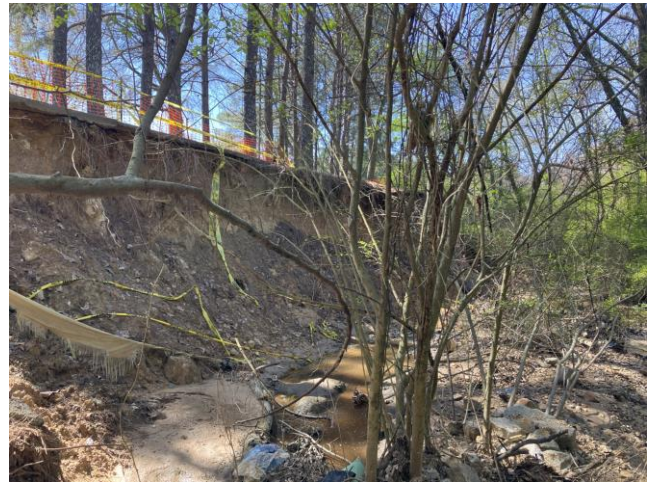
Photo 2: 10'-high eroded bank along greenway, creating public safety hazard, facing downstream
