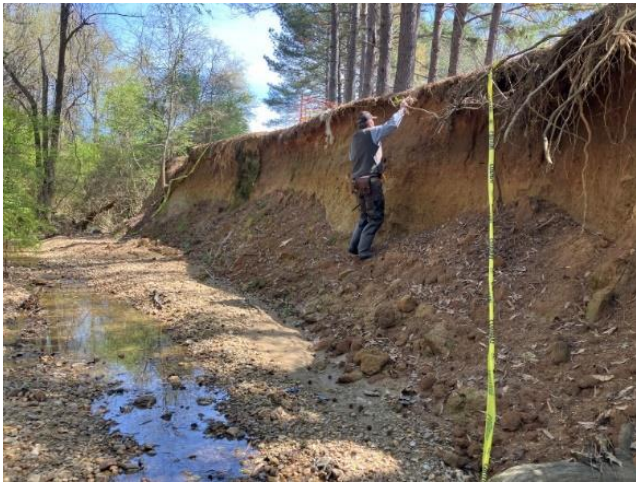
Photo 1: 10'-high eroded bank along greenway creating public safety hazard, facing upstream
